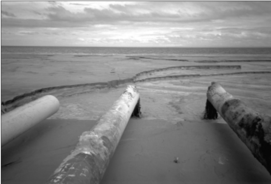
Marcopper tailings pipelines emptying into Calancan Bay, Philippines.
