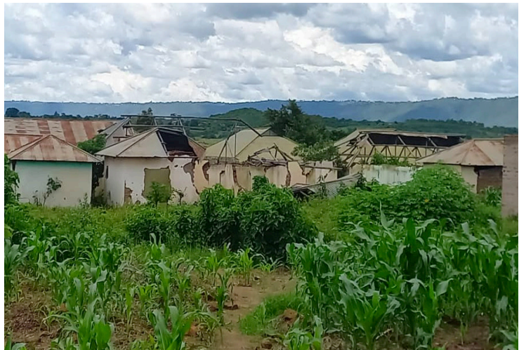
Photo: Houses assessed between 2012-2014 now falling apart in Kewanja Village as villagers wait for compensation. November 2023. (MiningWatch Canada)
