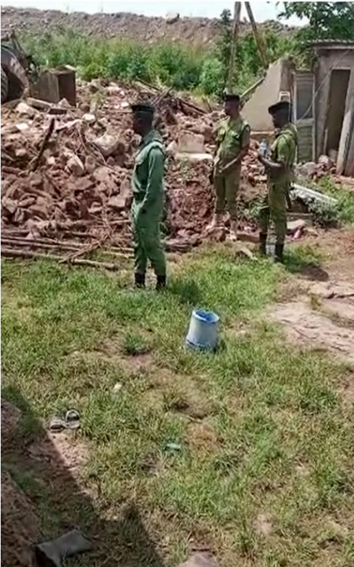
Photo: Police overseeing bulldozing of houses in Komarera Village. December 2022. (Still from video with MiningWatch)
